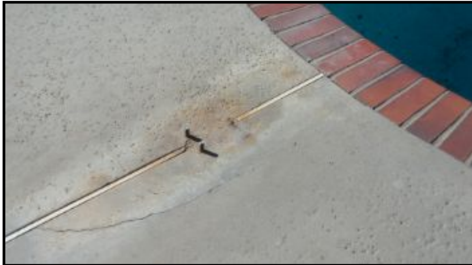
Trip hazard, bolts for diving board
